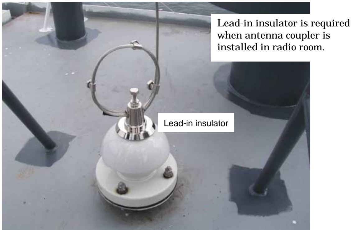
Fig. 3-5 Antenna lead-in insulator
