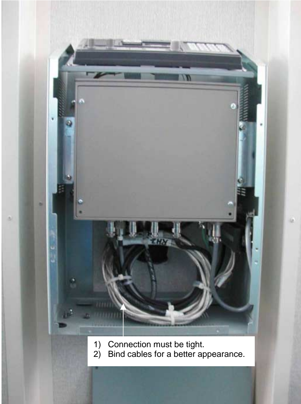
Fig. 3-26 Cables in VHF console
