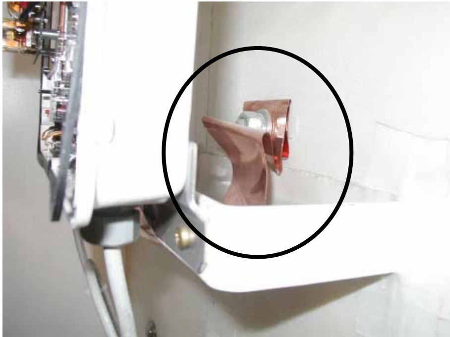
Fig. 3-10 Grounding antenna coupler
