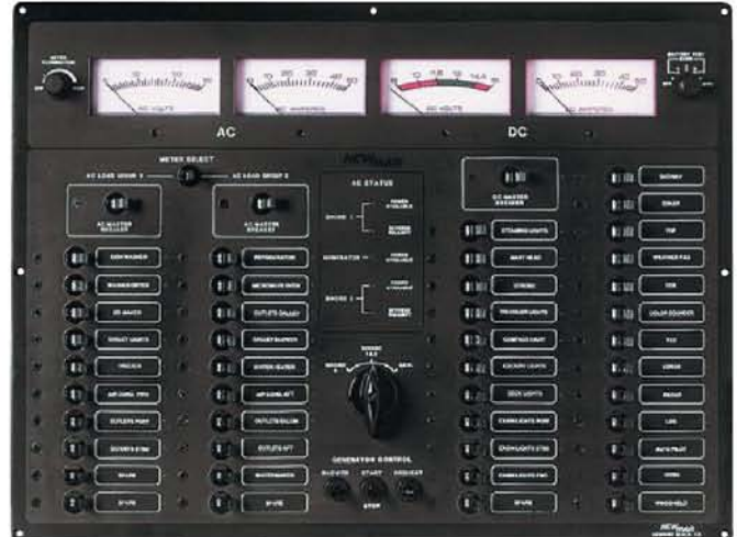
2 AC Load Groups + 10 Circuit, Dual Shore Power Selector Switch
